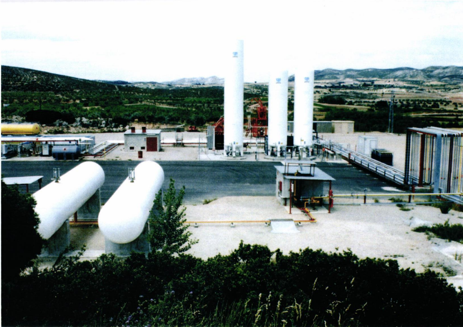
FIGURE 12 Injection Plant and Utilities Area
